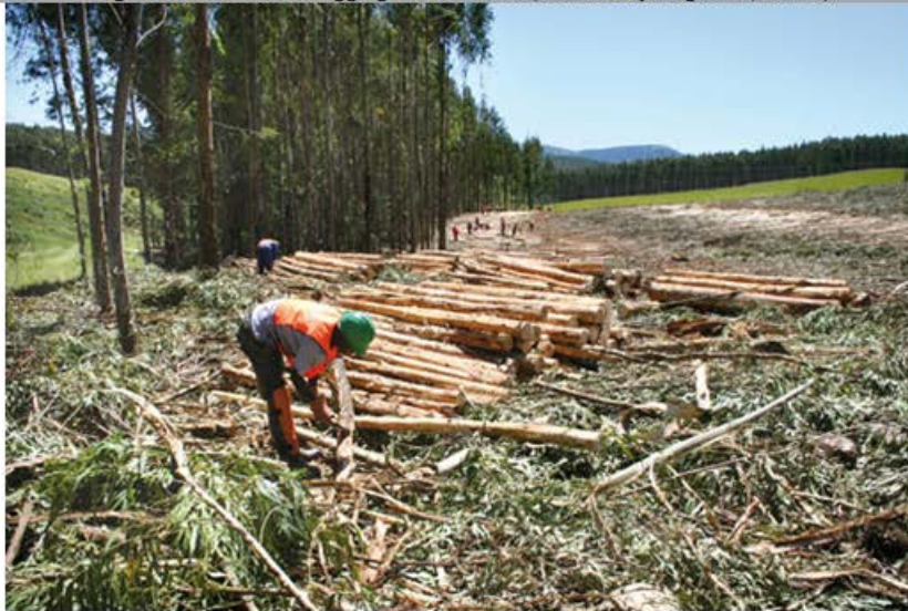
Fig. 7: Team of workers for lifting logs onto trucks (SA Forestry Magazine, 2011b)
