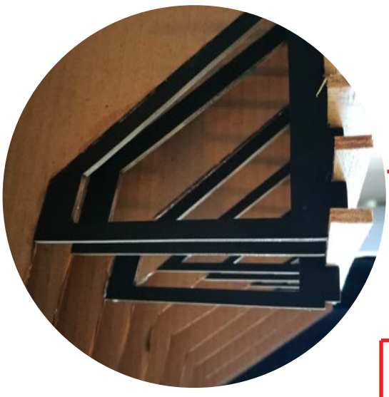
EARLY STRUCTURAL STEEL SUPPORT SYSTEM MOUNTED ON TOP OF RAMMED EARTH WALLS
