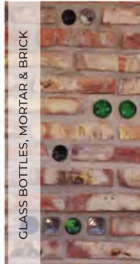
Gives ode to Familiarity within Melusi & promotes innovative ways for repurposing materials
