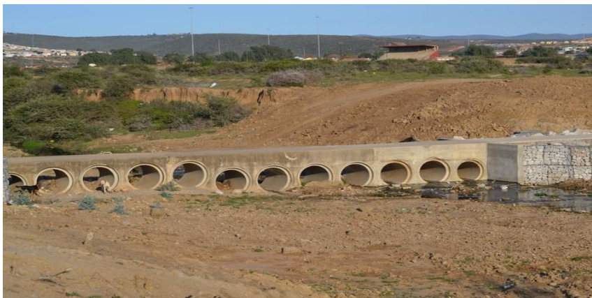
Figure 1.7.1 (b): Nelson Mandela Bay disappointing bridge (Mbovane, 2020).
