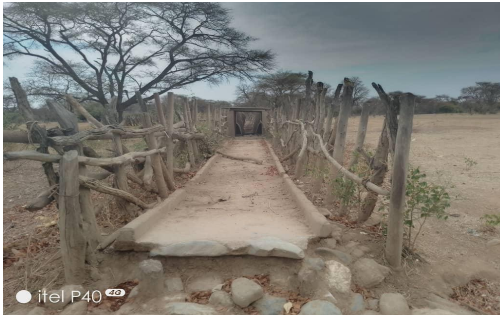
FIGURE 17: DILAPIDATED DIP TANK IN MURINGZAUVA (SOURCE: FIELD WORK 2022)
