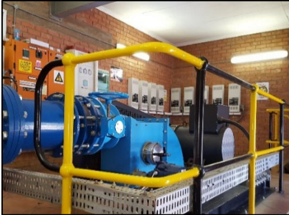
Crossflow turbine (96 kW) installed in bulk supply line, Bloemwater, SA
