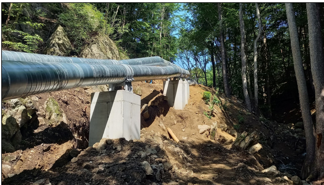
Figure 5: Two penstocks of Blansko small hydropower plant: DN300 (clean water from WWTP to small hydropower plant), DN400 (sludge from pumping station to WWTP)
