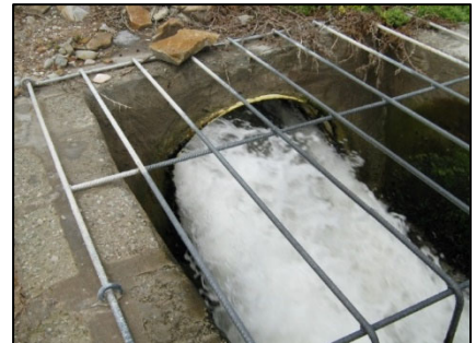
Potential 97 kW hydro installation at Abalone farm outlet, Gansbaai, SA
