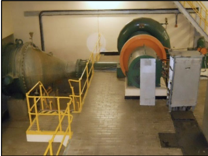
Francis turbine (600 kW) in the OFT Transfer Scheme, SA
