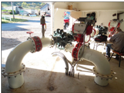
PAT (3 x 120 kW) installation on irrigation network, Utah, USA [7]
