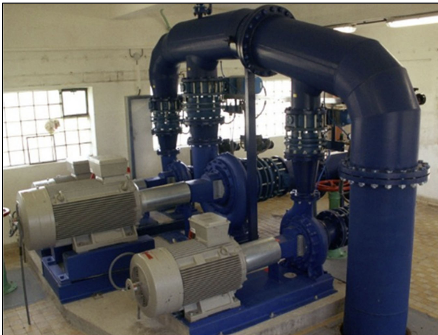
Figure 7: Small hydropower plant installed on raw water conduit in Vyšní Lhoty [14]
