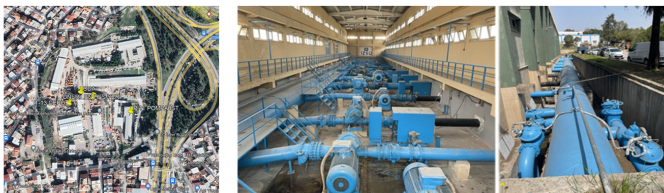
Figure 11: IZSU Karabaglar P11 Hydropower Plant (Türkiye)
