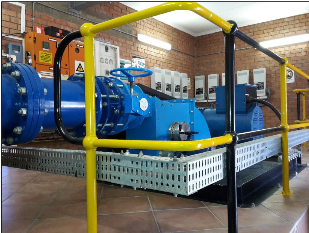
Figure 9: Brandkop Conduit Hydropower Plant (SA)
