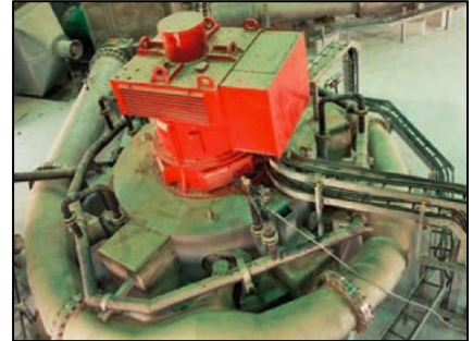
Pelton turbines (2 x 830 kW) Amman City, As-Samra plant (Jordan) [6]
