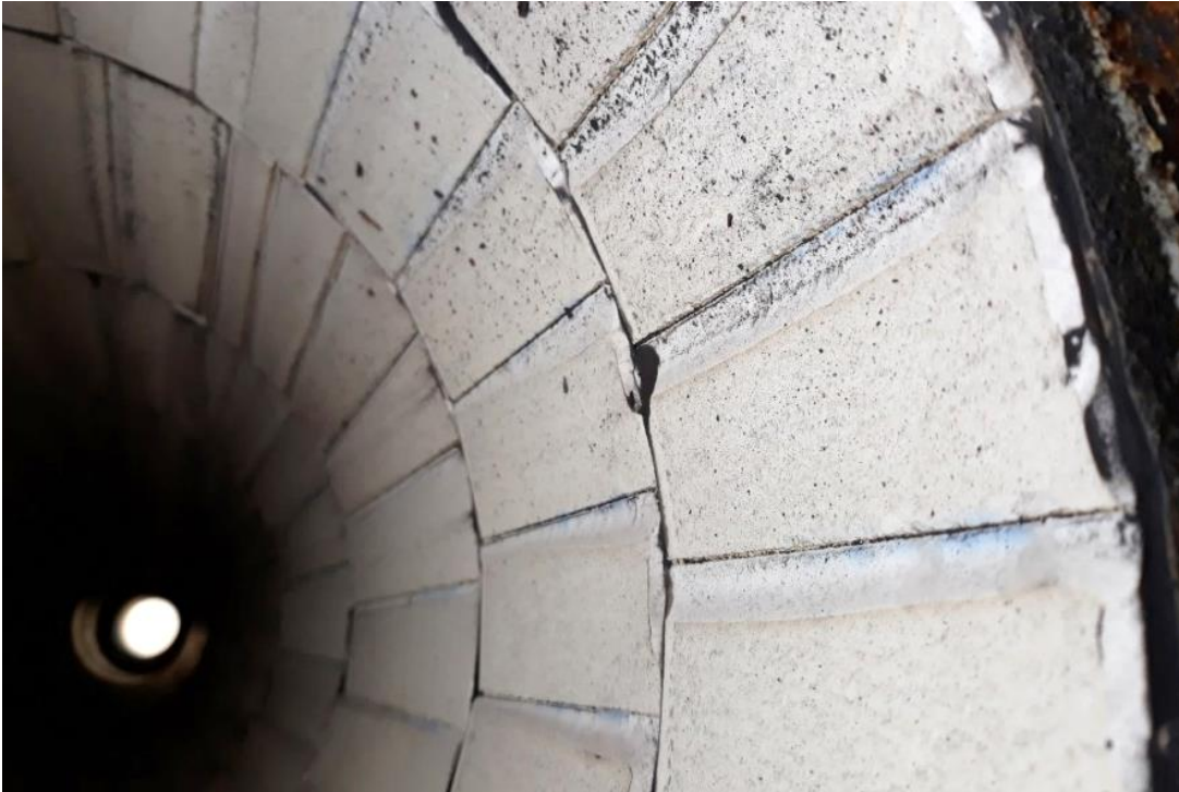
Figure G.5: Wear pattern on tiled part of overflow outlet of dense medium separation cyclone C510-20-0/BB-A/110 (RH) used for diamonds. The cyclone was in use for 6 months.
