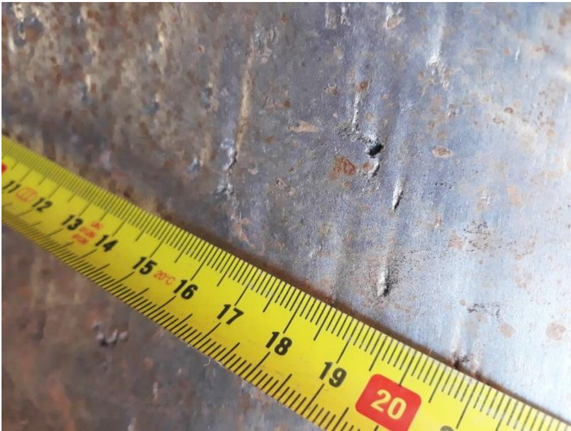
Figure G.4: Wear pattern at bottom of cone within dense medium separation cyclone C510-20-0/BB-A/110 (RH) used for diamonds. The cyclone was in use for six months.
