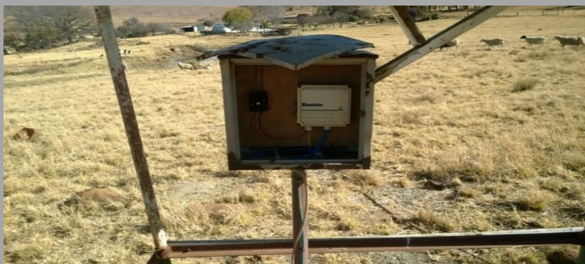
Electric panel not working, CMF Meeting, 2016
