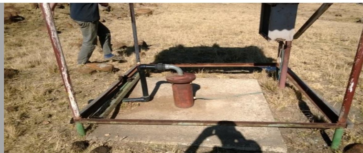
Vandalised Borehole, CMF Meeting, 2016
