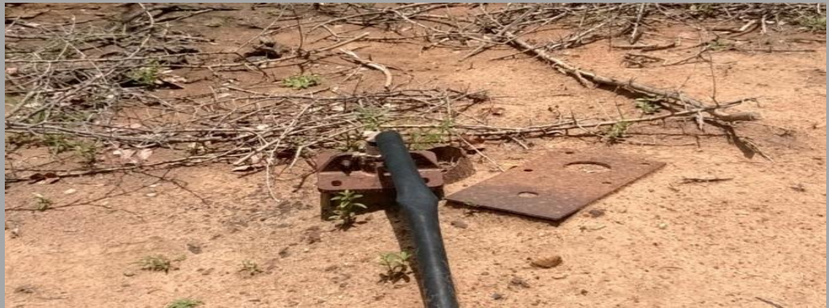
Vandalised Borehole, CMF Meeting, 2016
