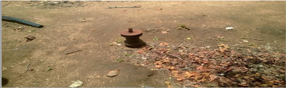
Vandalised Borehole, CMF Meeting, 2016
