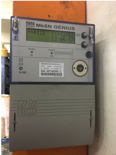
FIGURE 11: MOL SMART ELECTRICITY METER
