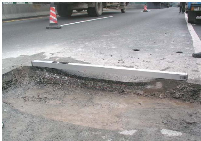
Figure 1. Rutting deformation of the cut edge.
