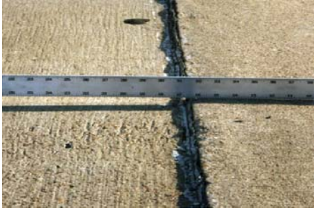
Figure 2a. Faulting destruction in cement concrete pavement.
