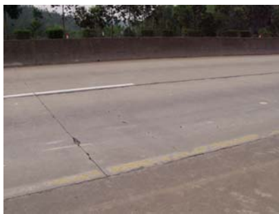
Figure 2c. Slab crack destruction in cement concrete pavement.
