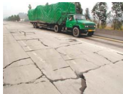
Figure 2d. Spalling destruction in cement concrete pavement
