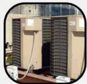
Fig 7.160 An example of an air-conditioning roof pack unit. ( www.daikin.com )
