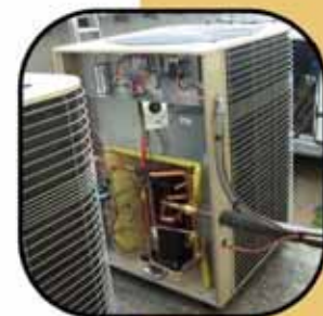
Fig 8.118 A ROOF PACK WITH THE ACCESS PANEL REMOVED. ( www.daikin.co.za )
