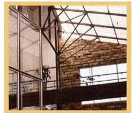
Fig 5.42A light steel roof structure carries translucent roof sheeting that allows diffuse light into the building's internal spaces. (Els, 2000)
