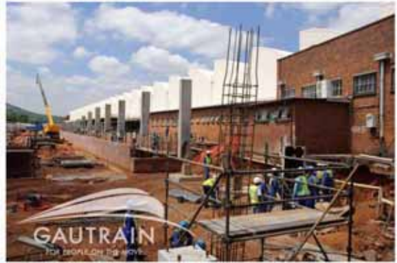
Fig 3.14 The New GAUTRAIN Station site during construction. The existing Merto Rail building can be seen in the background. (www.gautrain.co.za)
