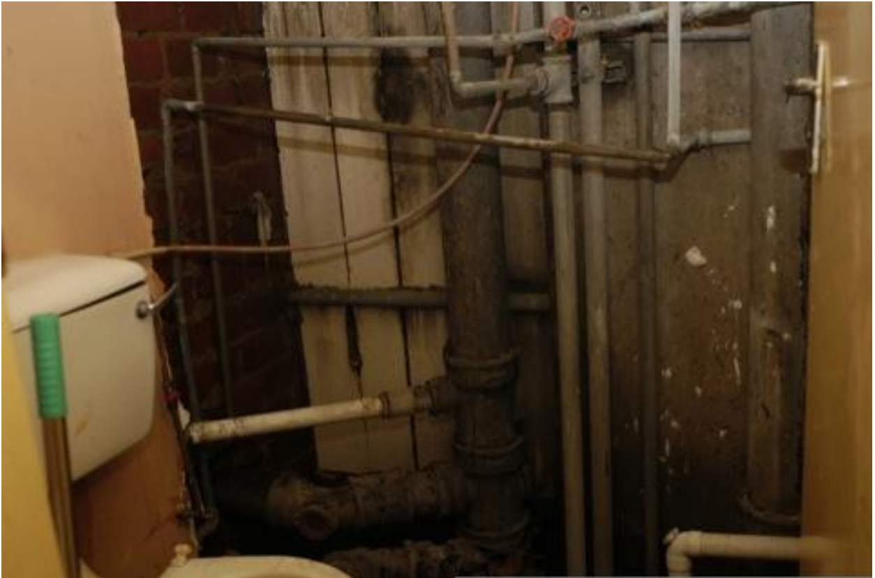
The walls of the buildings started caving in (Henning, 2008)
